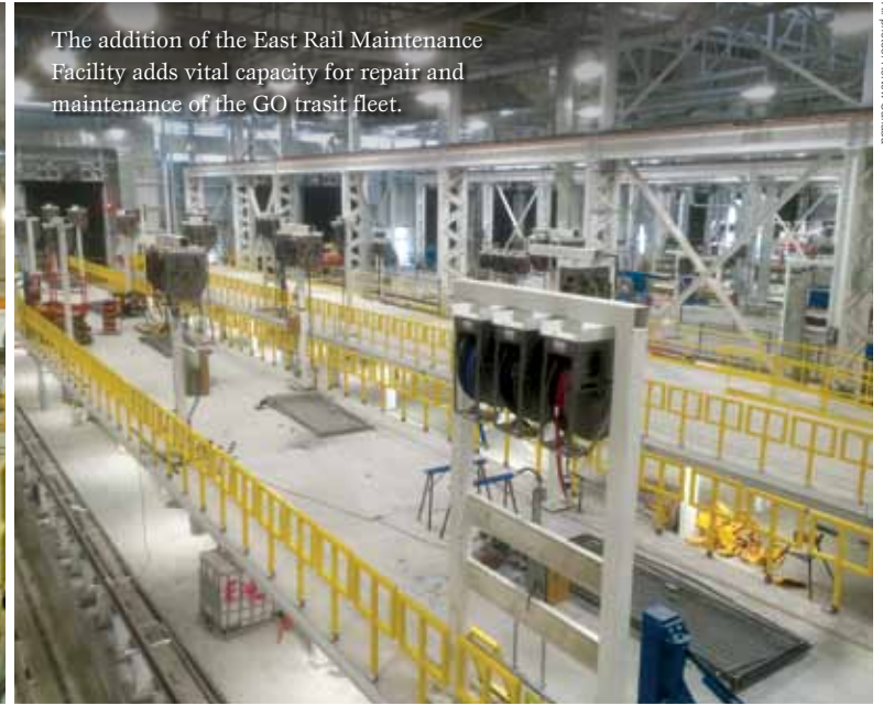
The ERMF infrastructure includes equipment that will support the electrification of the transit system.
