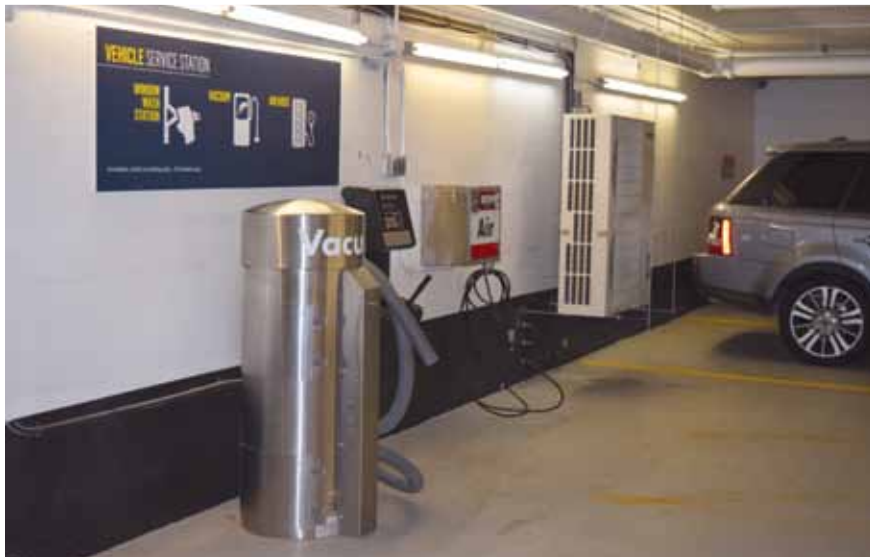
Green certification for parking structures includes installing things like carpool spaces, which encourage people to make green commuting decision.
