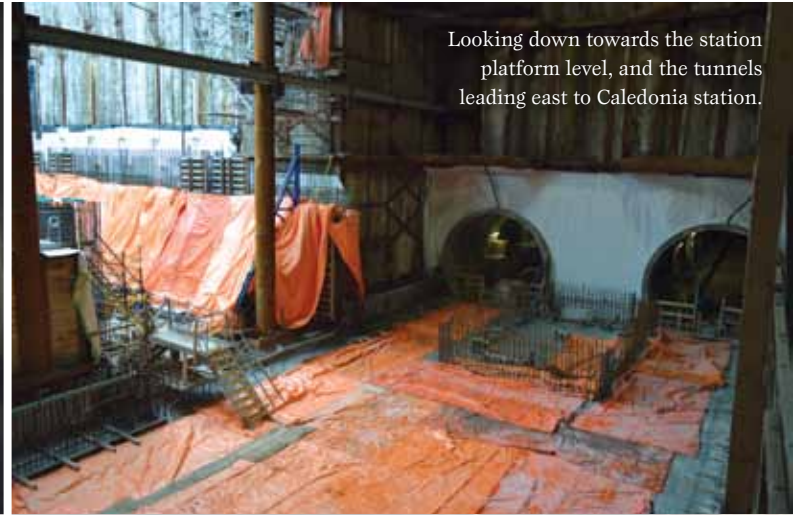
The tunnel to Caledonia has been formed, but track installation has not yet begun.
