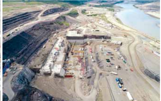
Credit: BC Hydro
